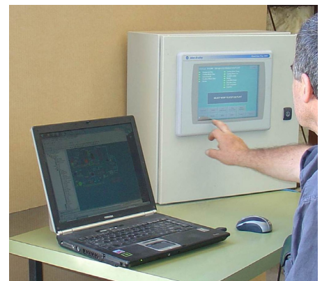
Remonitoring to allow monitoring of the CO 2 plant from the comfort of your own office or central control room.
