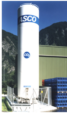
Vertical CO 2 storage tank
