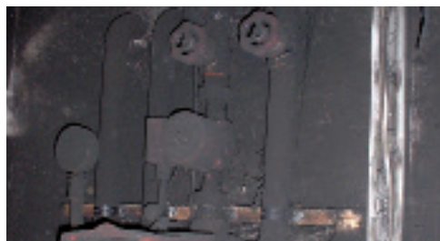
Fire damage before ...
